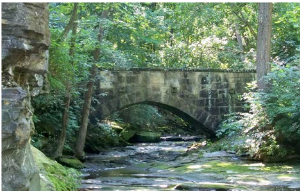
The stone bridge over Plum Creek using blocks of sandstone left over from quarrying was a Works Progress Administration project in the 1930s.
