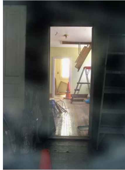
A peek through a window at the former West View Wesleyan Methodist Church in August revealed renovation work Clint Williams had initiated.
