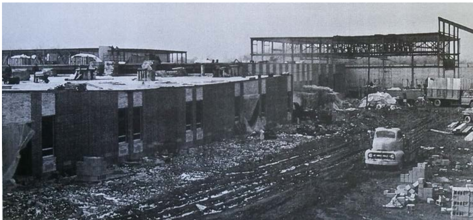
This photo shows the academic wing already under roof. The auditorium (right) and gym (rear left) did not have walls yet.
