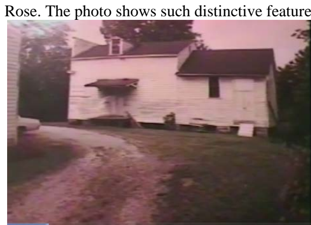
Another photo of the Granary from a Grand Pacific Junction video shows its deteriorated condition prior to renovation. Photo courtesy of Clint Williams
