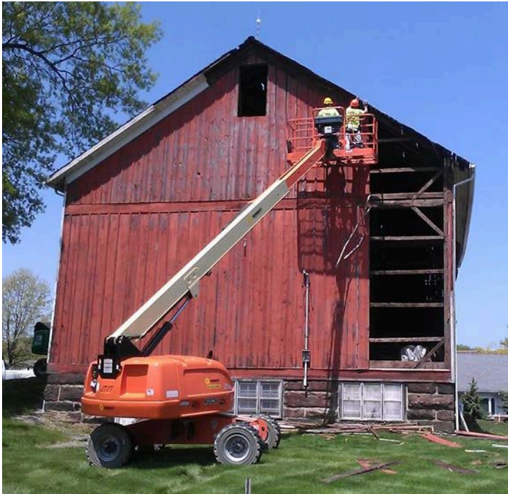
This photo from May 19, 2014, shows the beginning of the dismantling of John Hall's 1880 barn.
