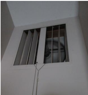
This fan prevents the attic from getting too hot.
