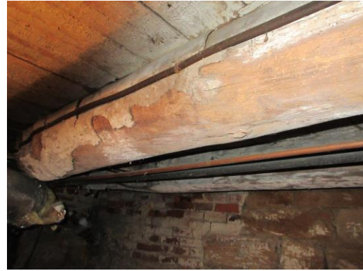
This is old crossbeam in the basement still has bark on it.
