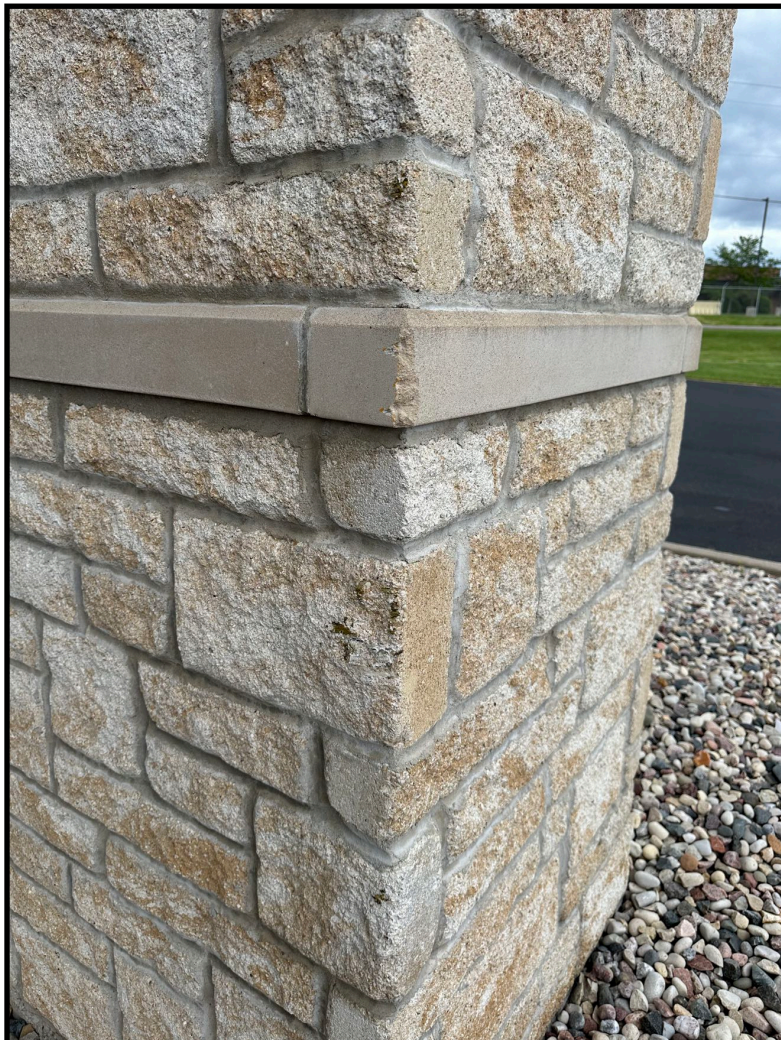
Pictured to the left the pillar with paint scrape marks.
