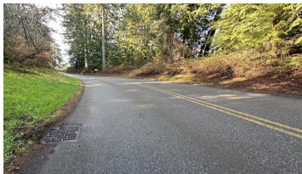
Thickened edge with Catch Basin is planned for LIP-5 (picture location Fairgrounds Road)
