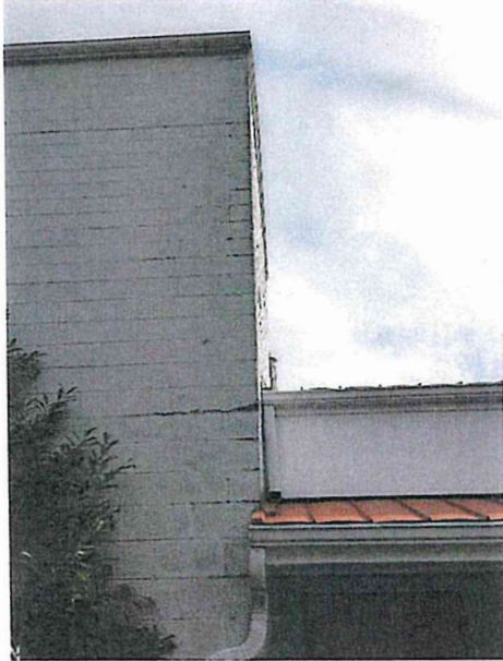
Figure 1 – Vertical Cracking (North Wall)
