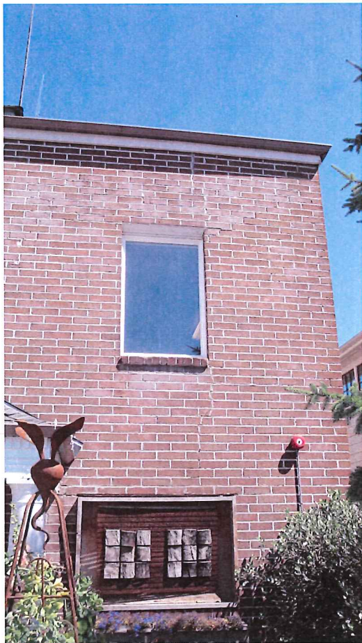
South Elevation – Typical Veneer Cracks
