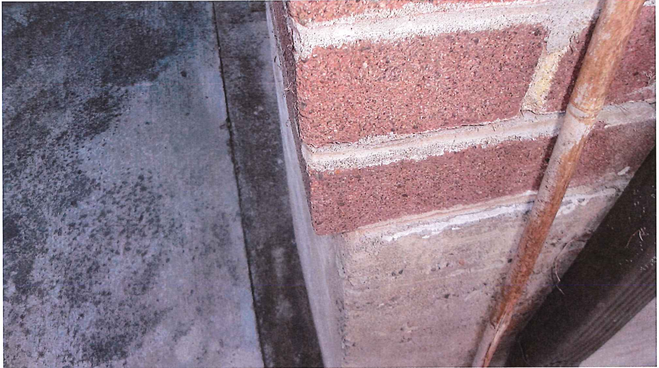
Northwest Corner – Veneer/Stemwall Misalignment
