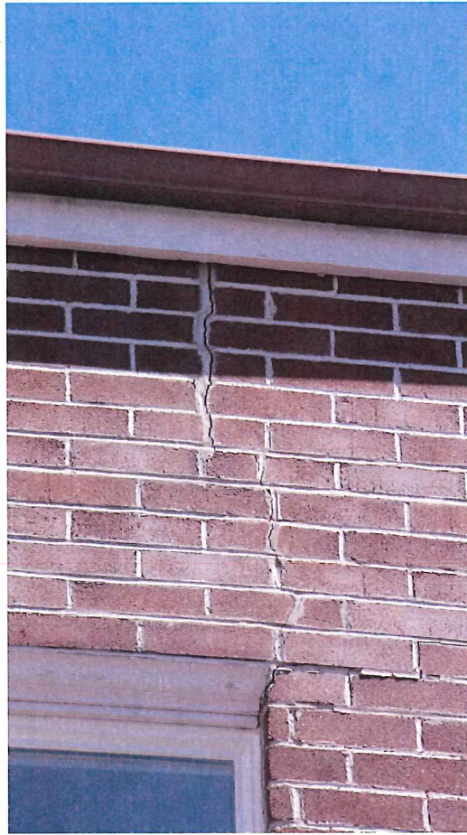
South Elevation – Previously Repaired Crack
