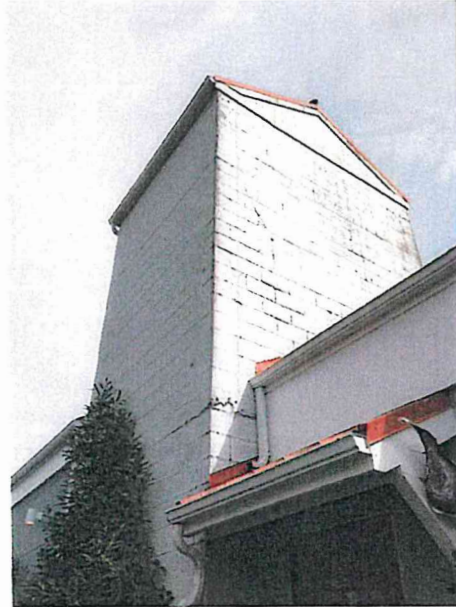
Figure 2 – Vertical Cracking (West Wall)
