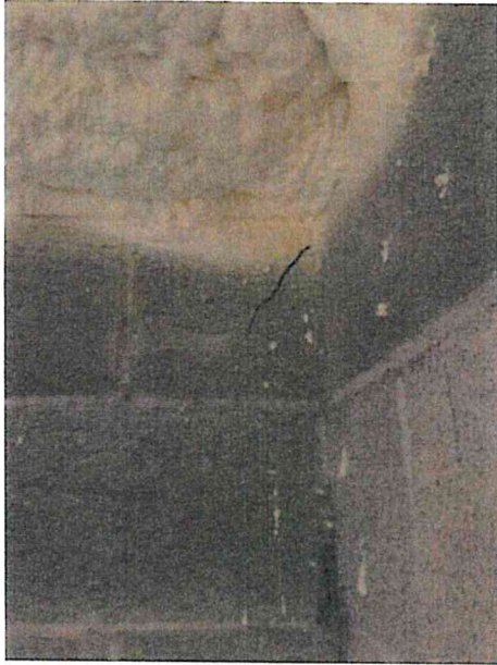
Figure 9 – Two Directional Crack
