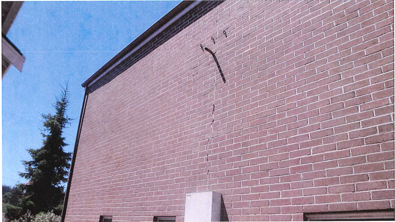
East Elevation – Veneer Crack
