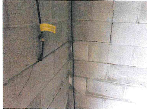
Figure 6 – Horizontal Cracking (South Side)
