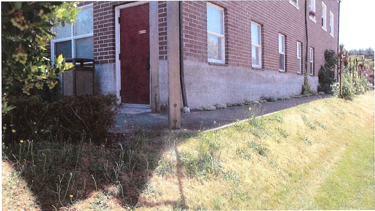
Northwest Corner – Back Door is Discontinuity in Stemwall
