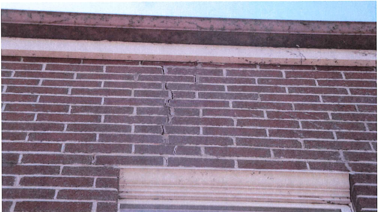
North Elevation – Veneer Crack
