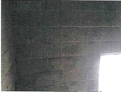
Figure 5 – Horizontal Cracking (North Side)
