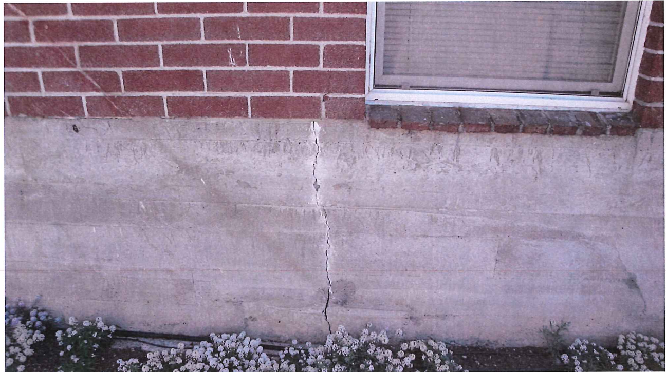
Northwest Corner – Stemwall Crack with Lateral Displacement
