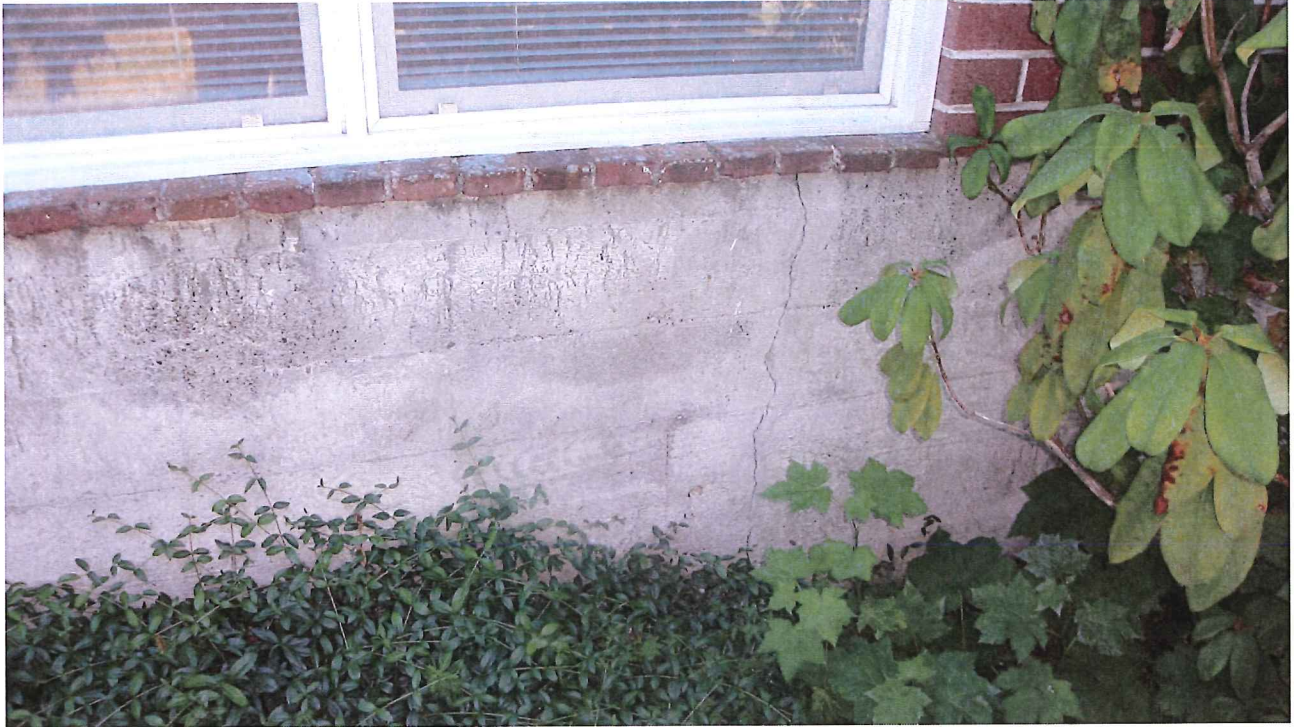
North Elevation – Stemwall Crack
