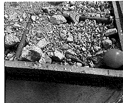
Photo S-20 [Swing Span] South pier protection cell, filling sinking, cracked weld on HSS bracing, looking south
