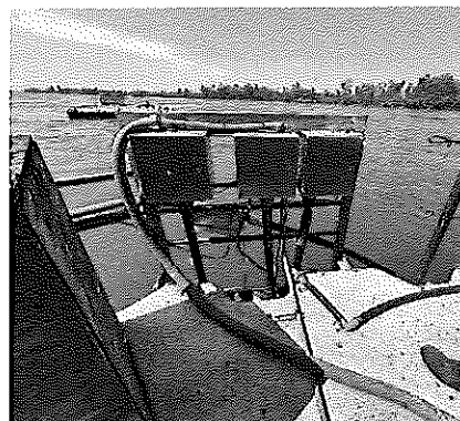
Photo E-10 [Pivot Pier] Submarine cable enclosures
