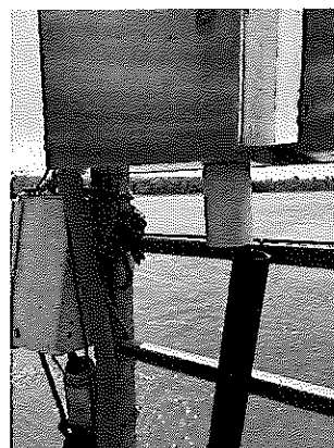
Photo E-11 [Pivot Pier] Duct cable coming loose
