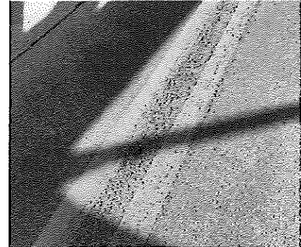
Photo S-01 [Span 4] Minor popouts at center line of bridge, looking west
