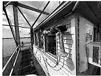
Photo E-16 [Operator's House] Air horn
