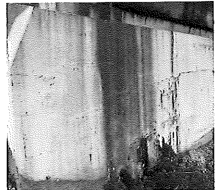
Photo S-19 [East Abutment] West face of East Abutment, hairline cracks
