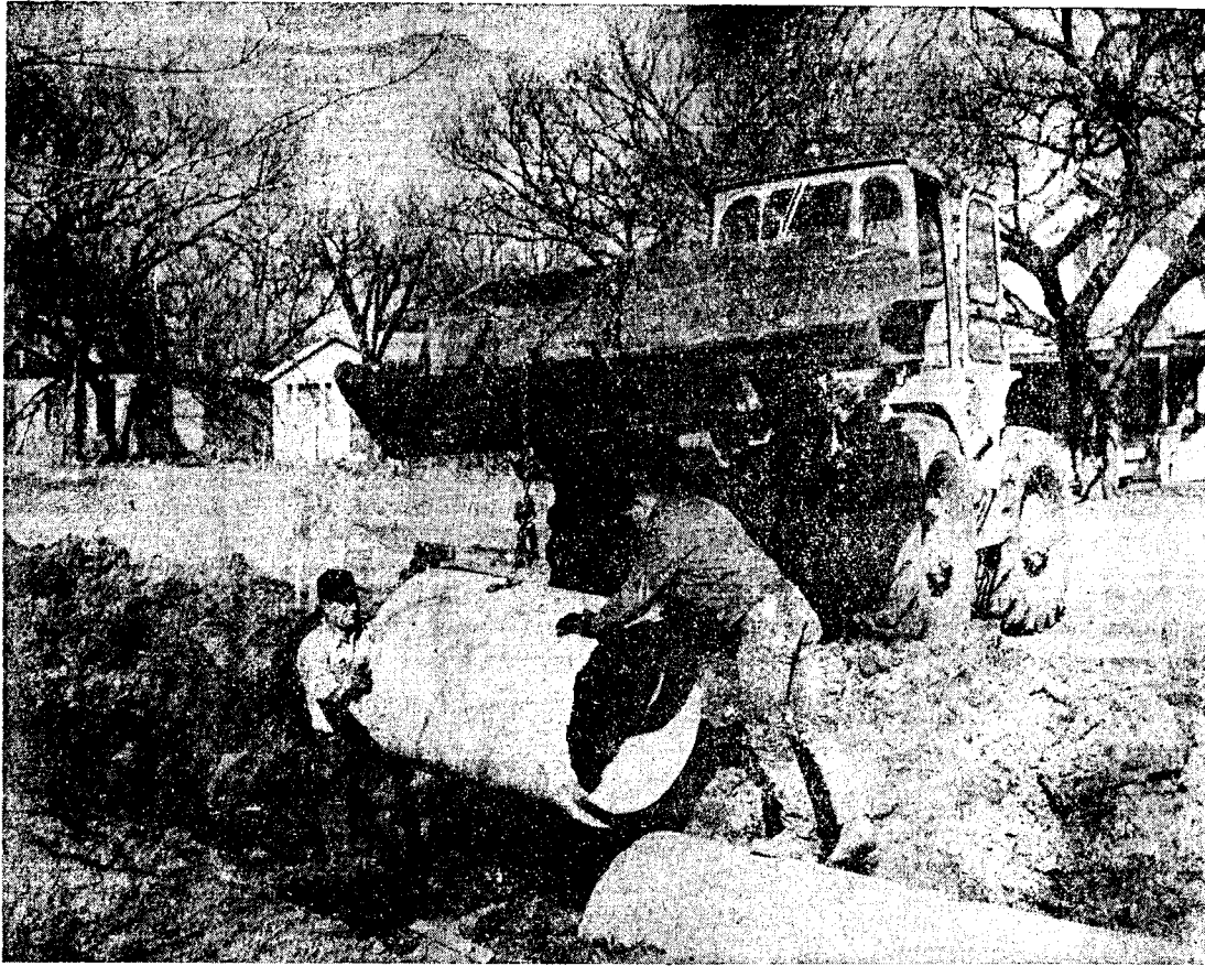
AN OPEN DITCH NO LONGER —City Public Works Department employes swing a big drainage tile into place in the storm sewer on Second Street just east of the viaduct and when the project is complete what has always been an open ditch will be a covered and tile-drained storm sewer. The 30-inch tiles are made right in the City shops during slack time in the winter, by city employes resulting in a great saving to the city on cost of the project. When more tiles are completed the storm sewer will be tied in to the other storm sewer under the viaduct. In this photo guiding the tile into place are Bob Stortz (left) and Tom Fisher (right). Scoop lift operator on the job was Cecil Dale and Roy Sidders was truck operator. (Blade-Empire Scan-a-graving.)
