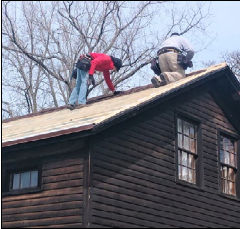
Old wooden shakes on the historic 1851 Richardson-Jakway House continually presented problems. The wooden shakes were replaced with a steel roof designed to appear like the historic roof.
