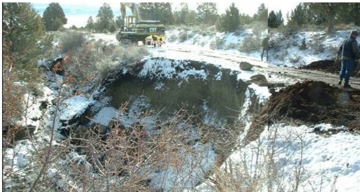
Figure 4-41 County Road 9 Washout, April 12, 2005
