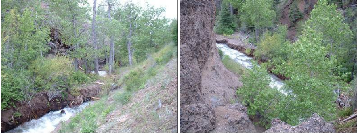
Figure 4-32 2005 Erosion near County Road 11
